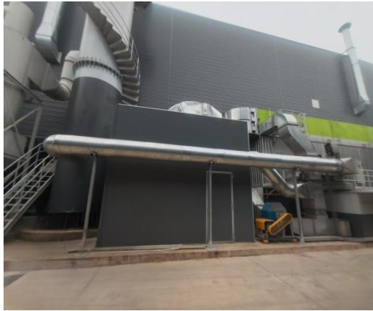
DA015 纸盒过滤+活性炭吸脱附+催化燃烧
